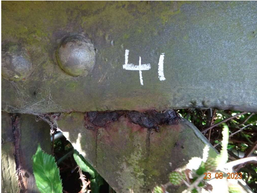
Figure 25: Typical example of corrosion found on the Northern truss. Diagonal bracing member (Defect 41)
