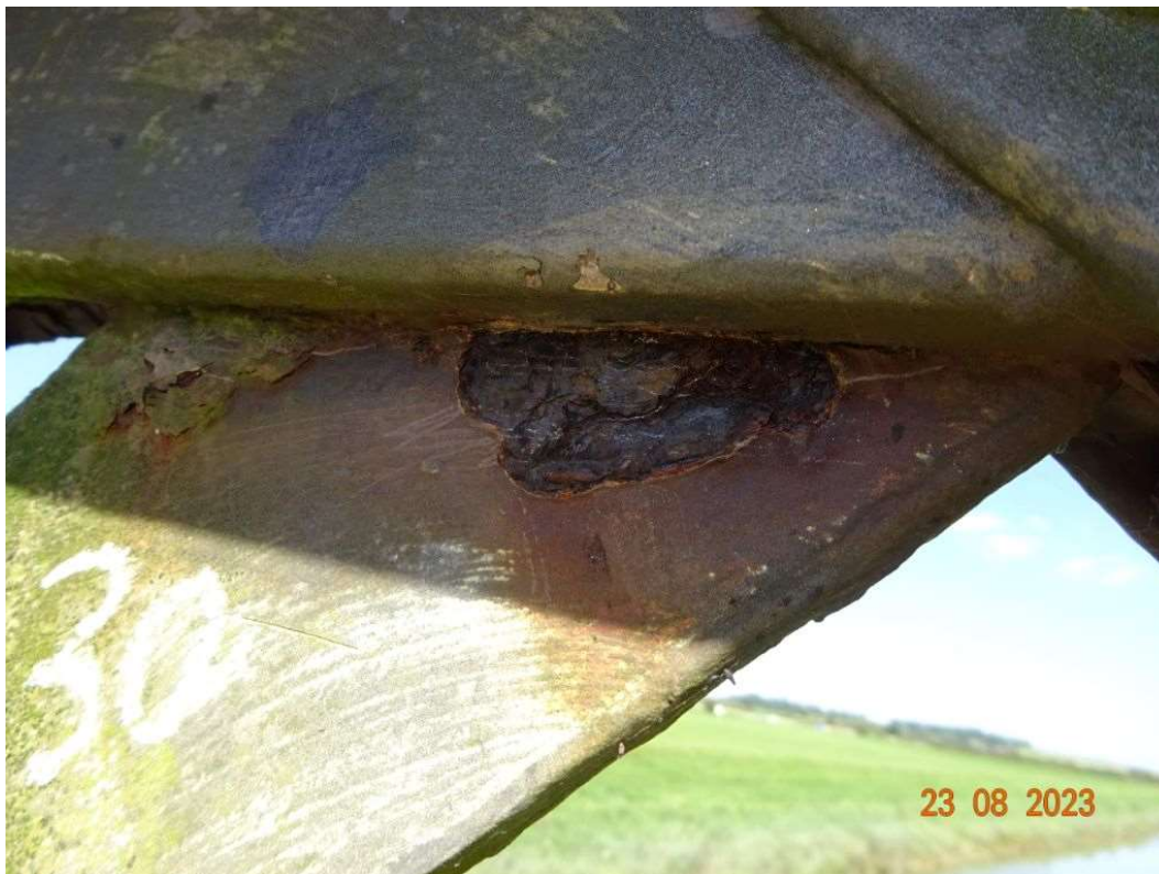
Figure 26: Significant pitted corrosion of diagonal bracing member – Northern truss (Defect 30)
