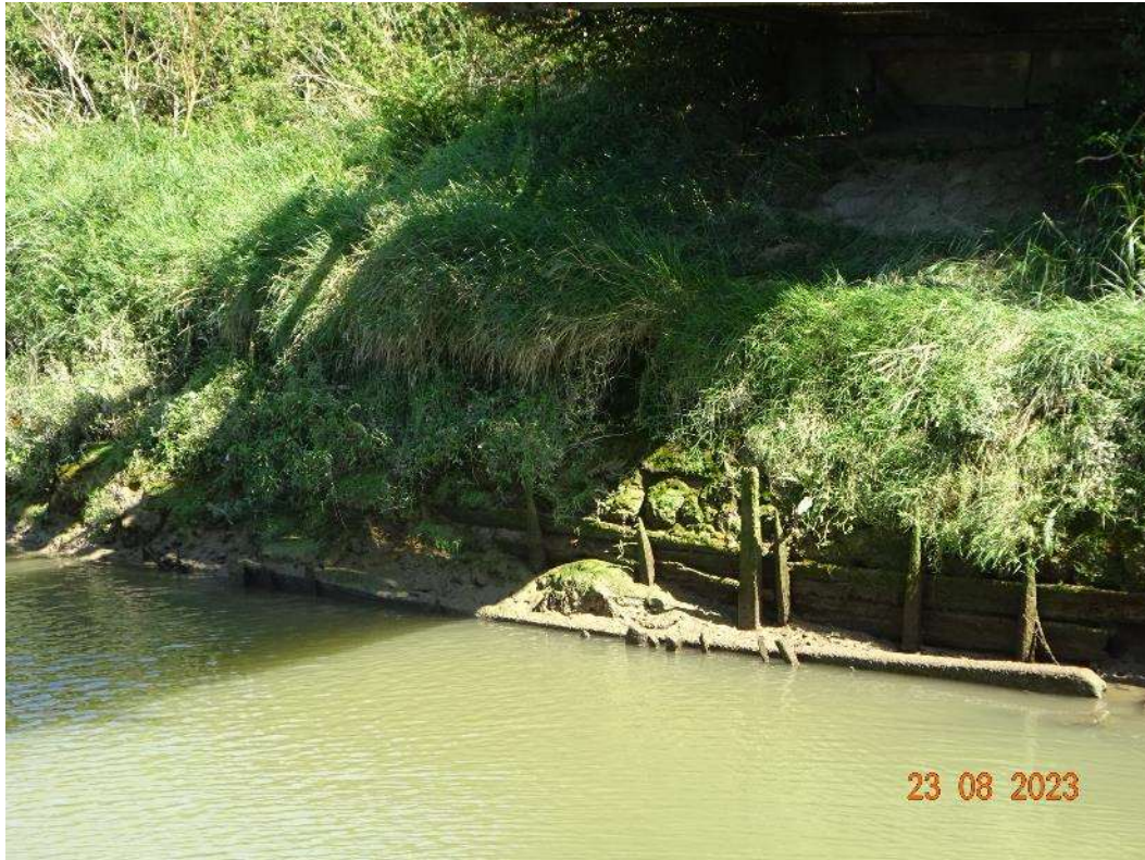
Figure 23: Deteriorated timber wall to east embankment.
