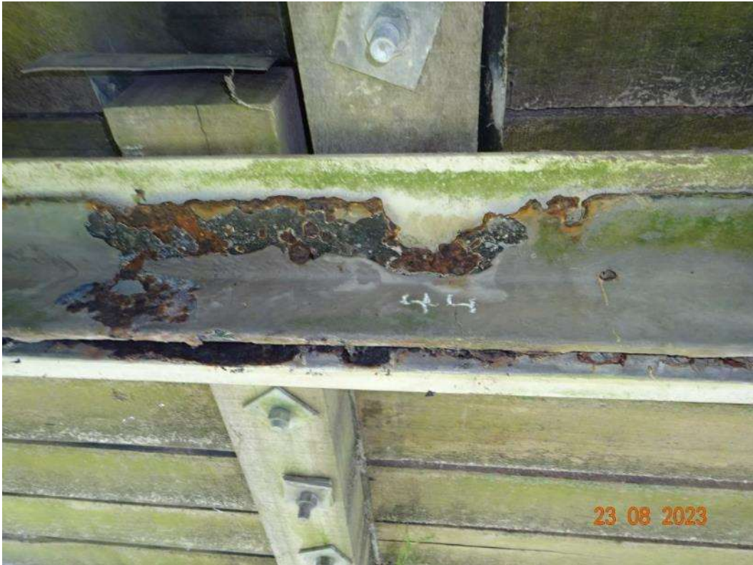
Figure 17: Sectional loss to underside of outrigger (eastern end).
