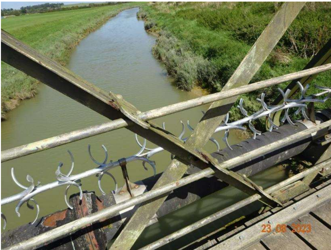
Figure 20: Slight paint losses to parapet railing.
