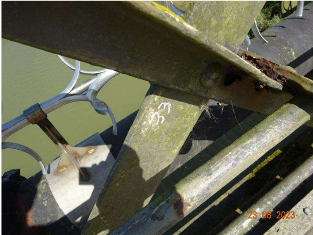
Figure 21: Minor surface corrosion to parapet railing.
