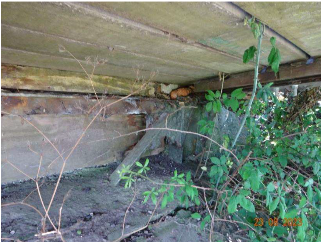
Figure 18: Transverse crack to concrete (east).
