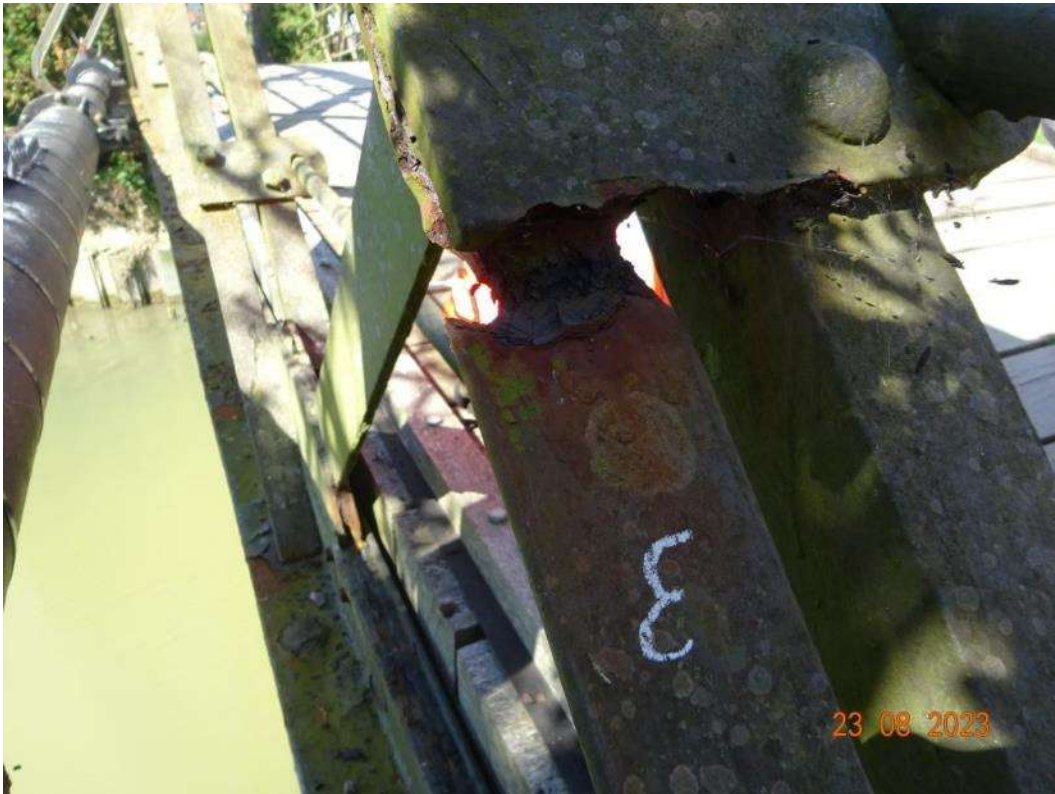
Figure 5: Disintegration of diagonal bracing (external plate, south)
