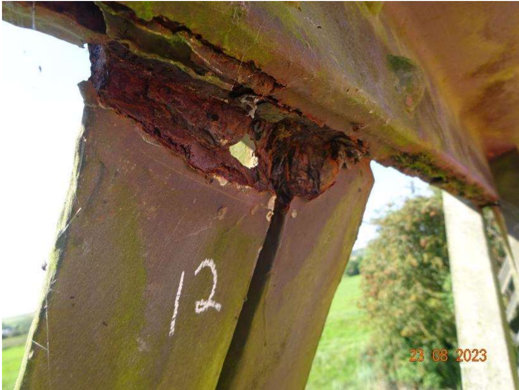
Figure 15: Loss of thickness and perforation to outrigger (south).
