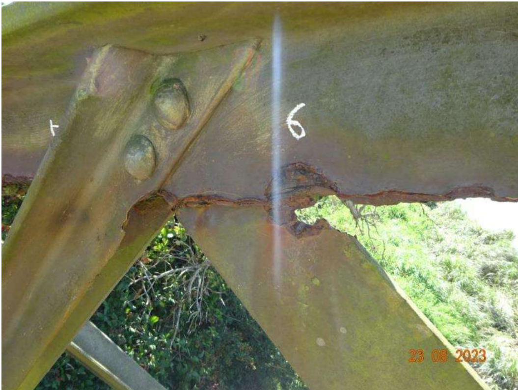
Figure 3: South Truss - View of disintegration corrosion to top chord and diagonal bracing (Defect 6)
