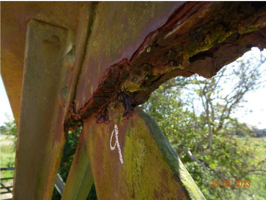
Figure 4: South Truss - View of consistent corrosion to top chord and diagonal bracing (Defect 9)
