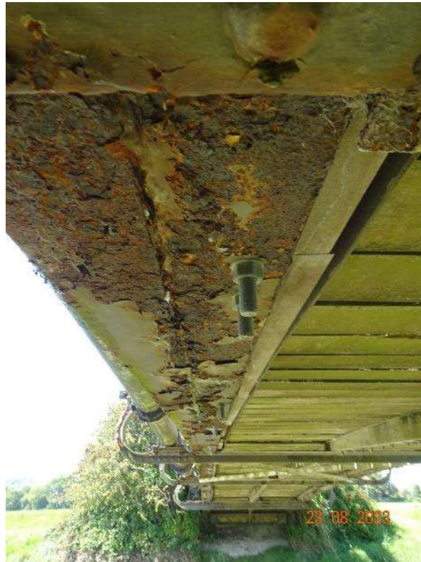
Figure 7: Severe pitting corrosion to bottom chord (south)
