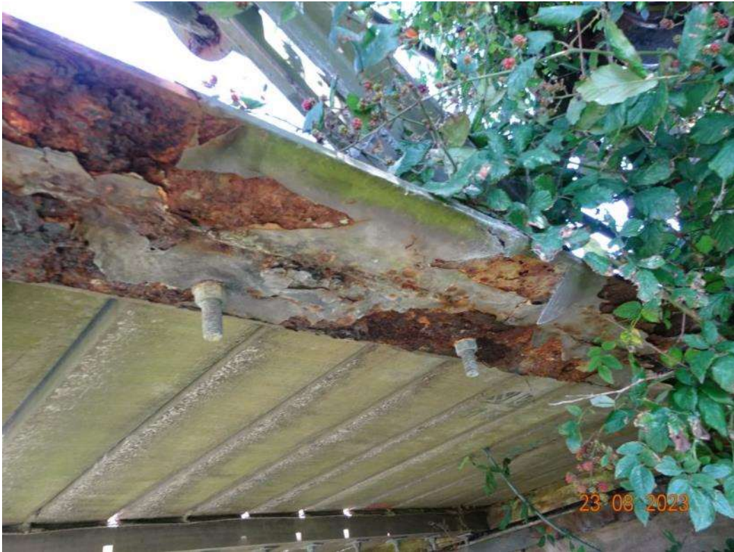
Figure 19: Significant paint loss allowing for corrosion to develop.
