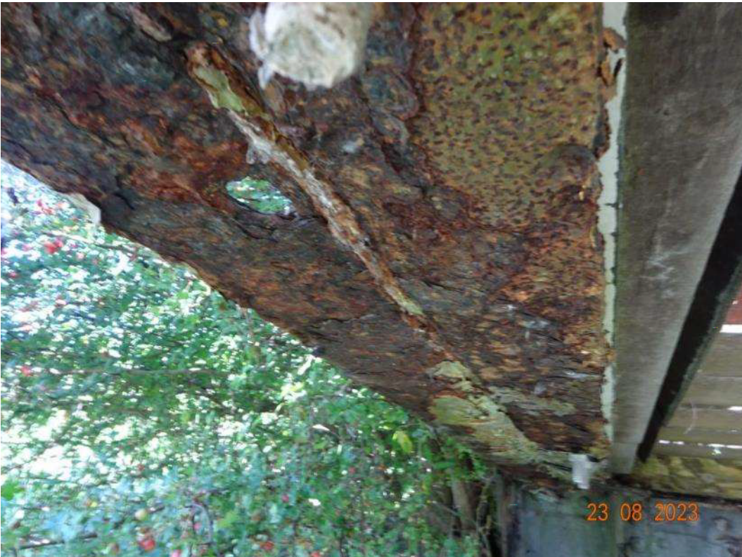
Figure 12: Disintegration to exterior plate of bottom chord (north).
