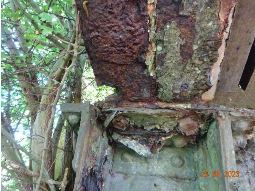
Figure 11: Disintegration to underside edges of bottom chord (north).
