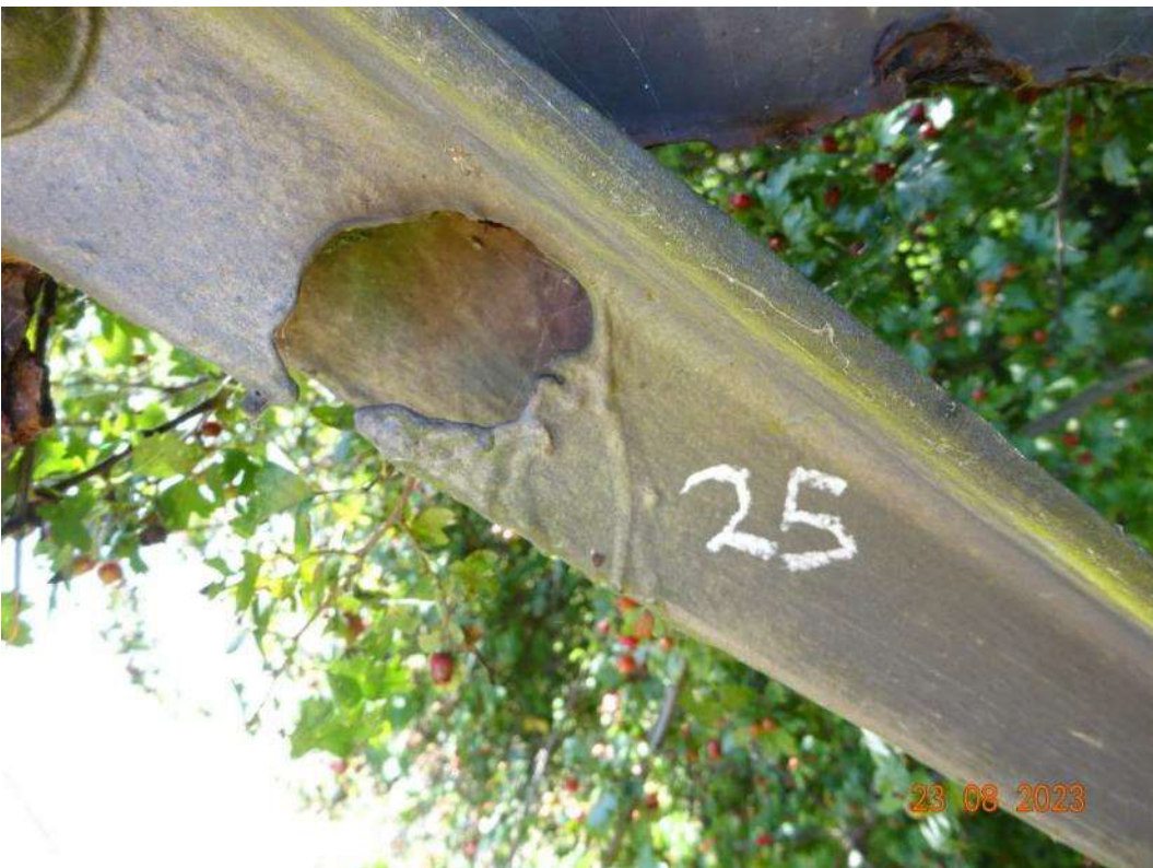
Figure 6: Disintegration (historic) of diagonal bracing (internal plate, south)
