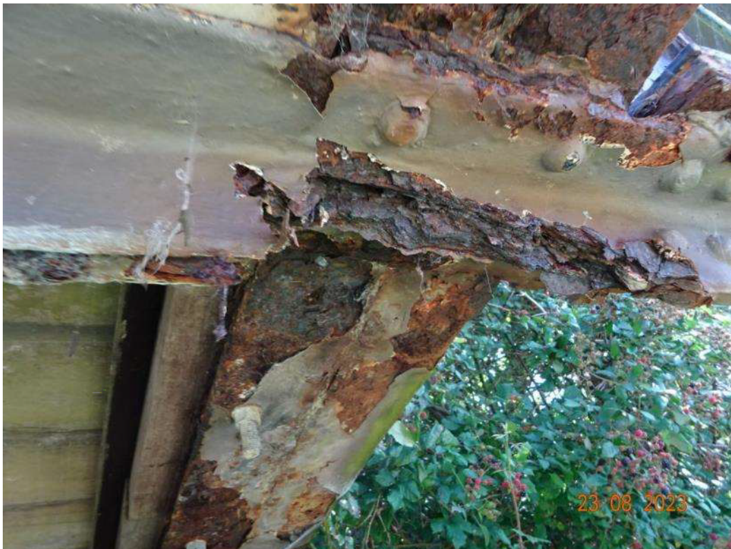
Figure 16: Sectional loss to underside of outrigger (photographed southeast).
