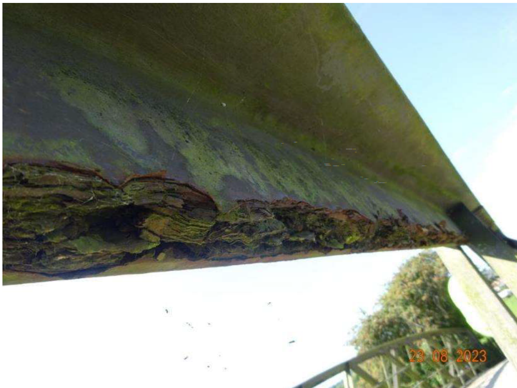
Figure 8: View of typical moder-major corrosion to underside of northern top chord
