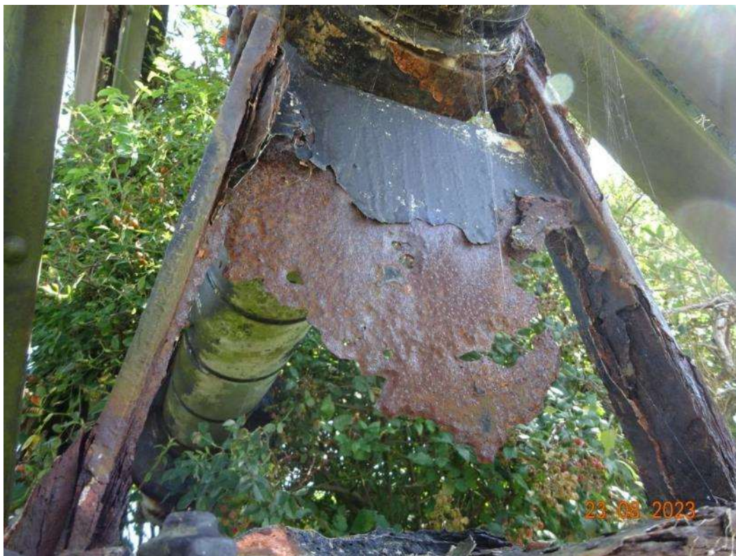
Figure 24: Disintegration of service pipe supports, pictured to south side.
