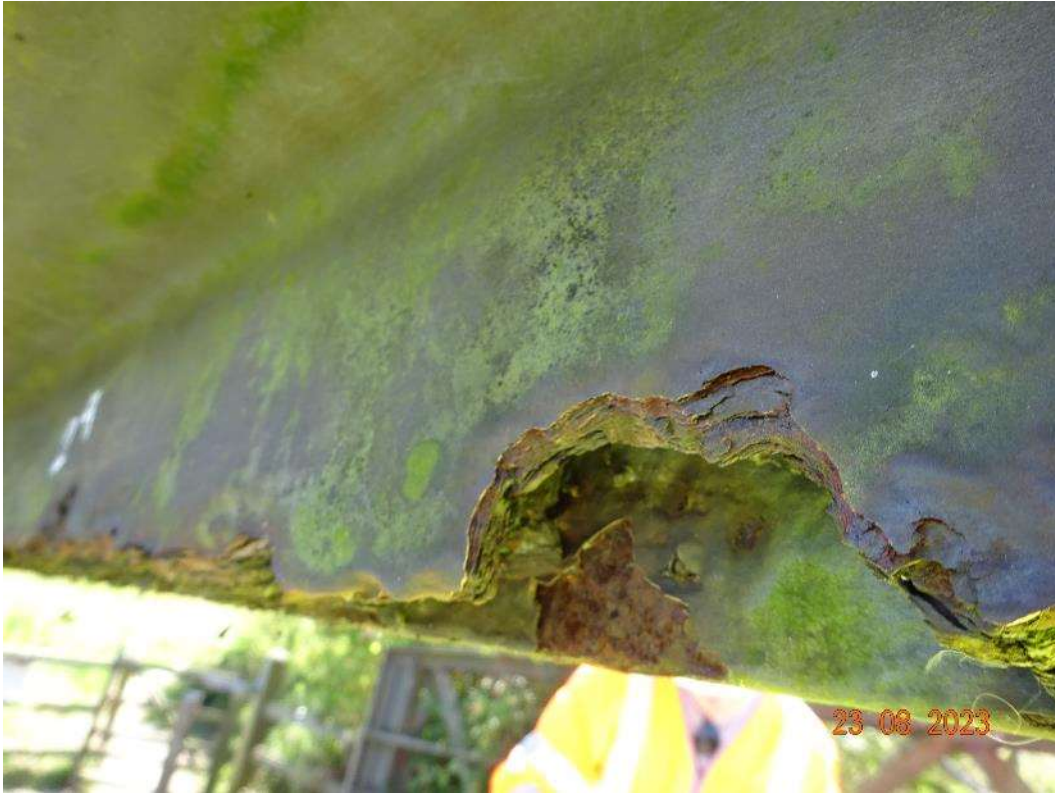
Figure 9: Major section loss to exterior member of top chord (north)
